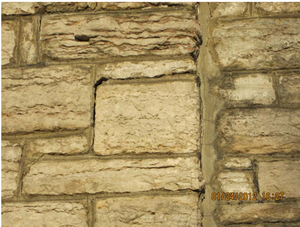
Section of exterior wall needing tuck-pointed.
