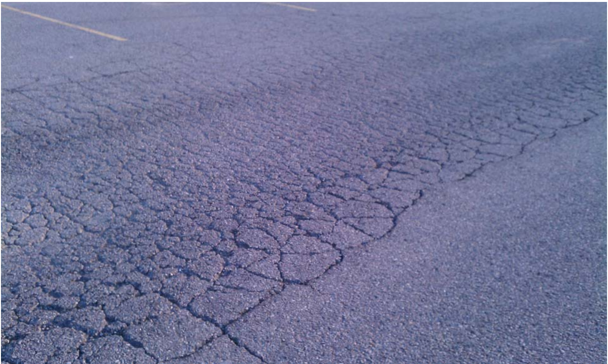
Many sections of the older parking and drive areas are in disrepair.
