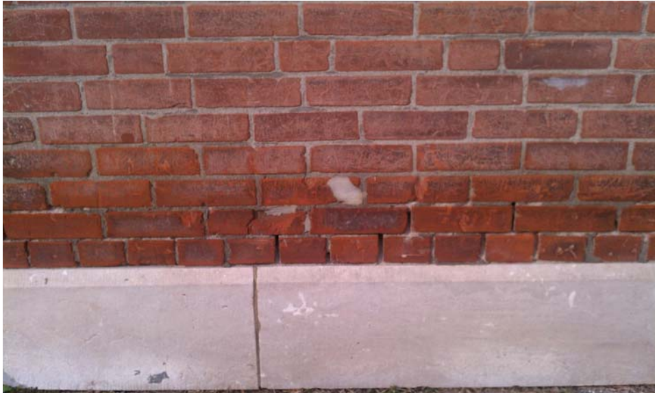
The brick needs tuckpointed.
