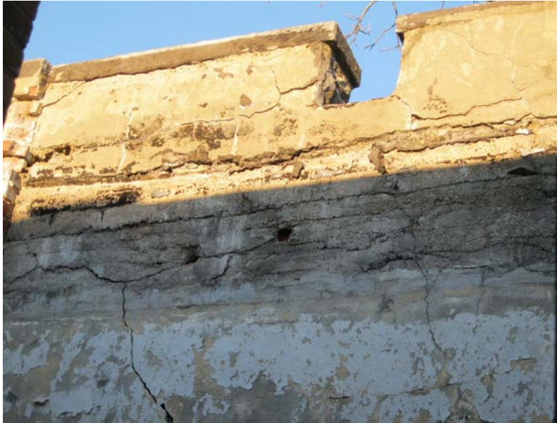
Interior wall needing mortar repair and paint repair.
