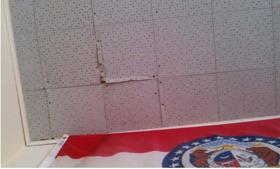
The ceiling tiles are sagging and need replaced.
