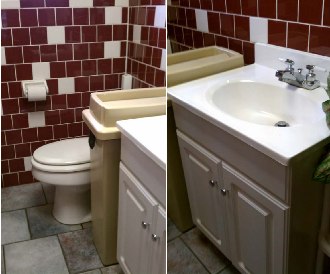
Restroom in Pro Shop, not compliant with accessibility standards: no grab bars at toilet, no knee room under lavatory, no 5' diameter turn around
