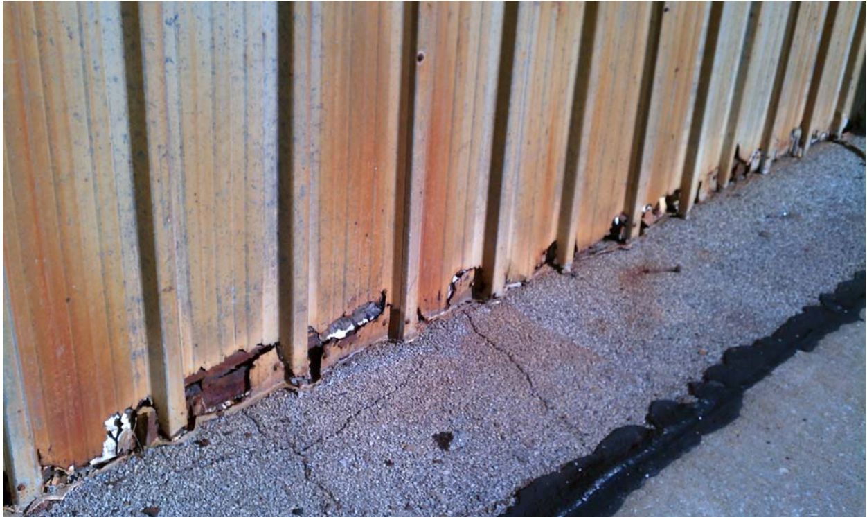
Damage to the metal building panels on the Corporate Hangars, caused by the runway ice melt.
