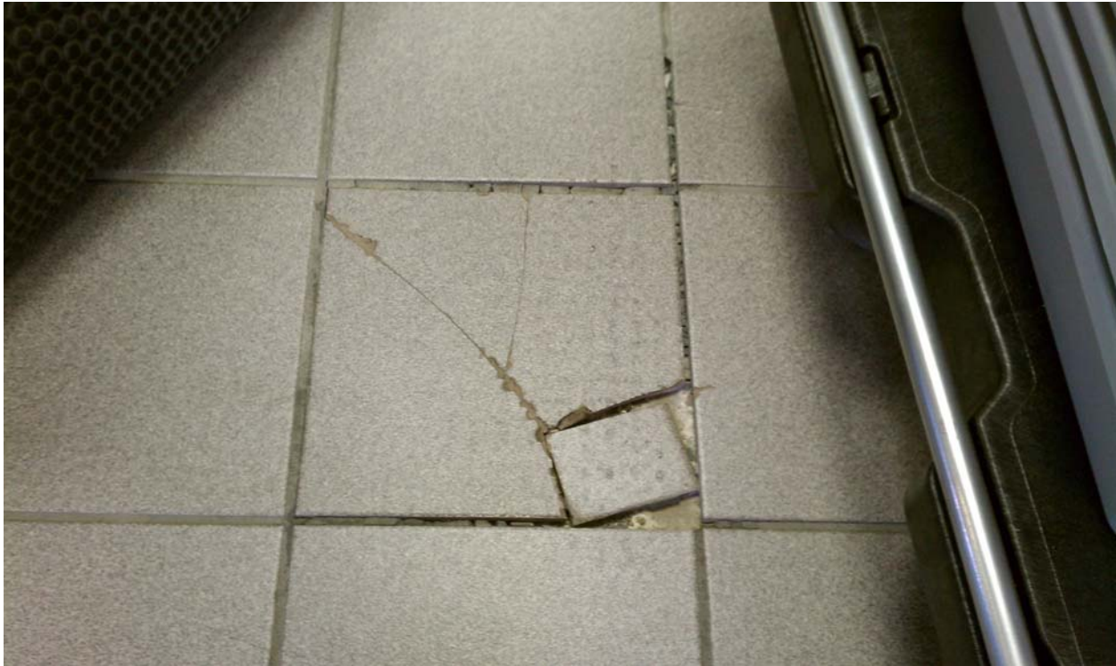
Cracking tile in the Terminal Building.
