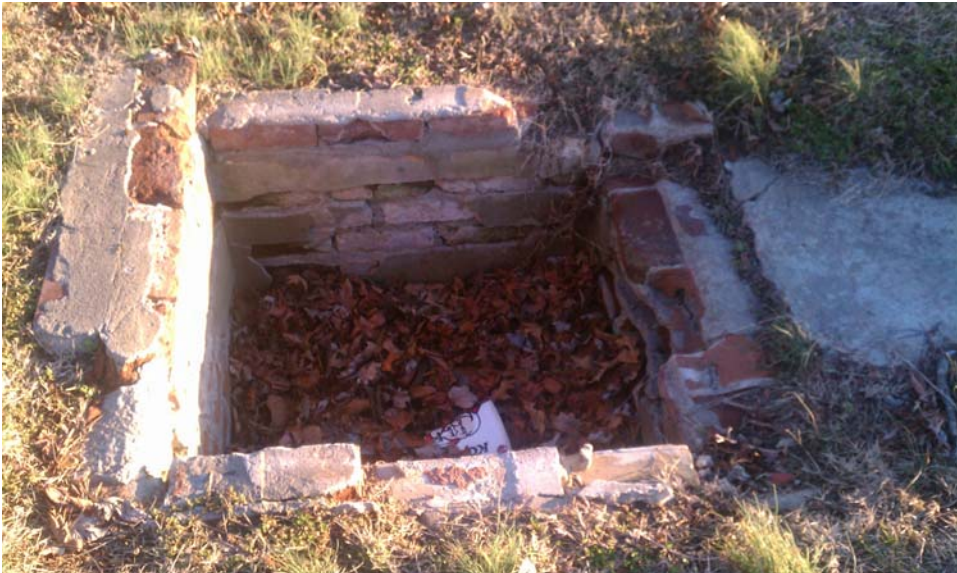
The cooking pit, that poses a trip hazard without the grate installed.
