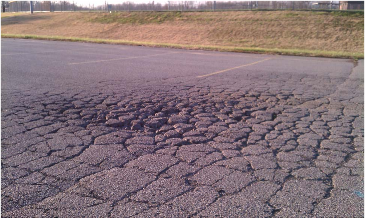
A section of parking lot paved in 1997 that has not been maintained. It will need milled and resurfaced.
