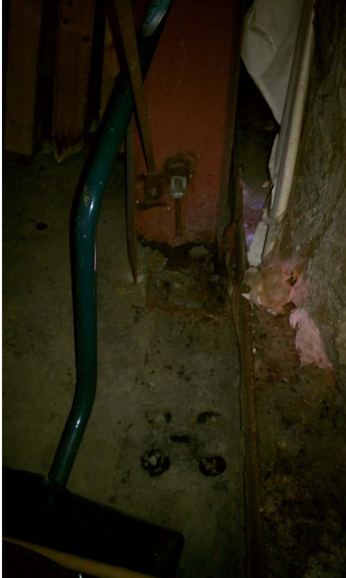
Deteriorated metal column in the Corporate Hangar. This column is no longer supporting the building.
