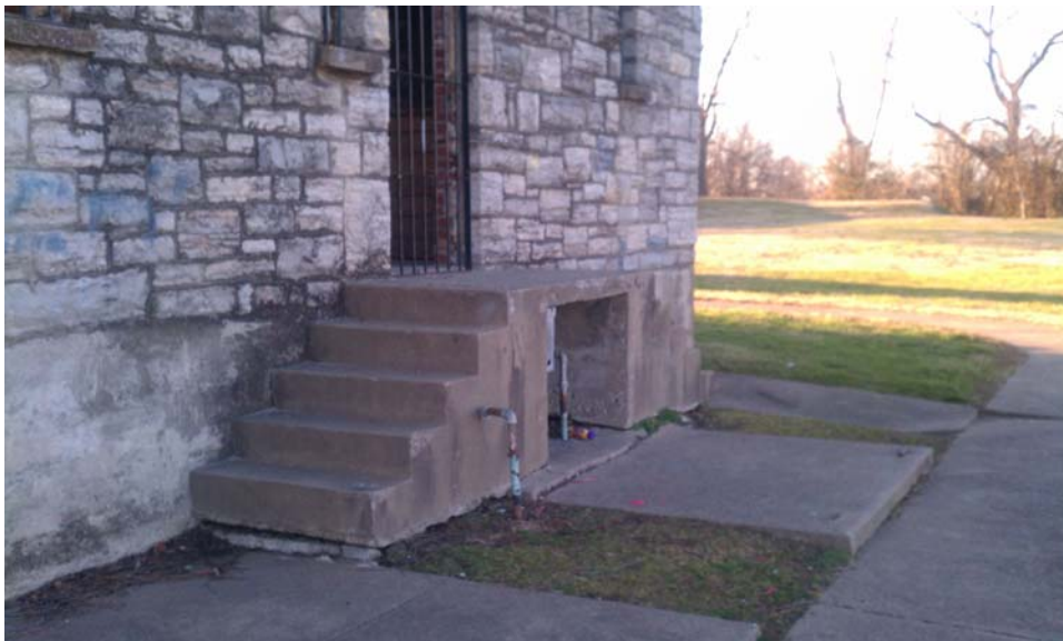
The stairs on the east side of the structure that need a handrail and guard installed to comply with the International Building Code.
