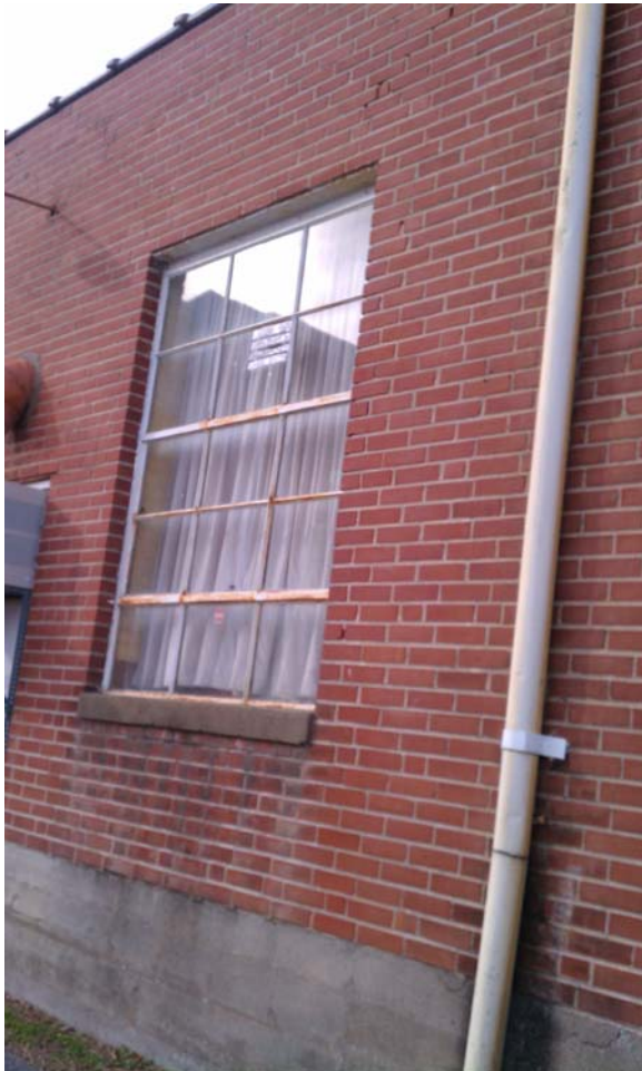
The brick also needs cleaned and resealed.
